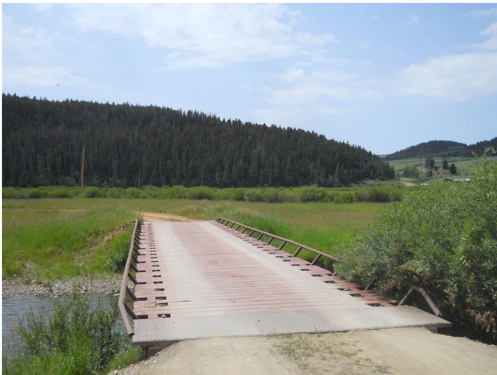
Figure 4.2b Modern Railroad Flat Car Bridge in the NW1/4 of Section 30, T12N R7E, View to the West.
